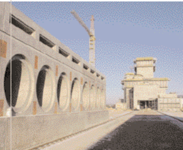
Construction of the new "dry" storage facility of irradiated fuels on the Chernobyl site.
