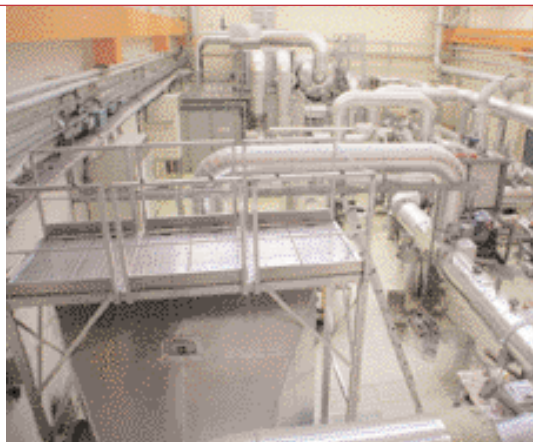
Starmania facility used to study the behaviour of containment and compartmentalisation equipment in case of fire.
