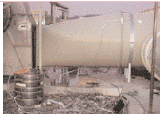
Canalised sampling of an odorous gas sample.
