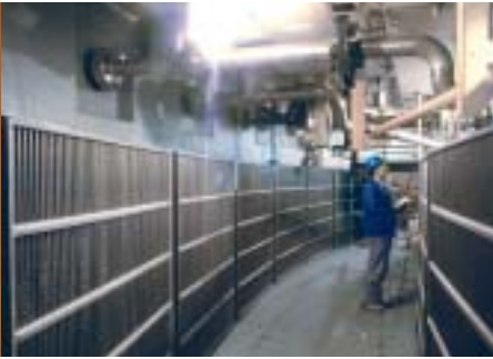
RIS sump, Civaux nuclear power plant (Vienne).
