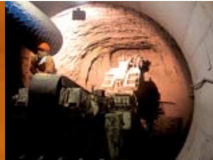
Excavation of the main gallery in the experimental installation at Tournemire (Aveyron) in 2003.
