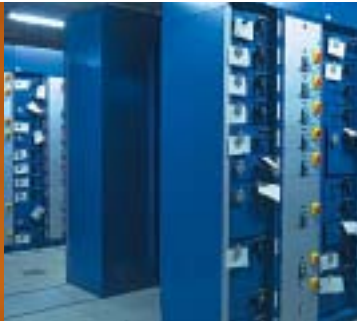
Locked-out electrical cabinets in the electrical building of plant unit 2 of the Civaux power plant (Vienne).
