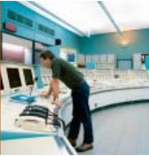
Agent at the control console in the Le Blayais power plant control room (Gironde).
