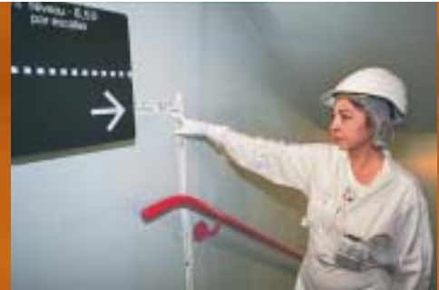
Floods in December 1999 inside the Le Blayais power plant: indication of the rising water level in the premises housing the spray system heat exchanger in the fuel building.
