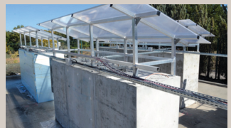
Installation ODE © IRSN/Gilles Bertin-Maghit
