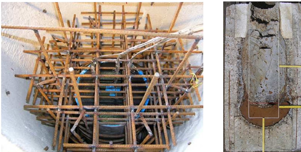
Figure 10: MOCKA 3.1 - View of the rebars before concrete pouring (upside-down) and post-test cut of the test section
